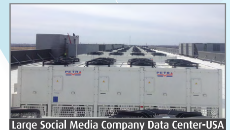
Large Social Media Company Data Center-USA
