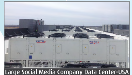
Large Social Media Company Data Center-USA
