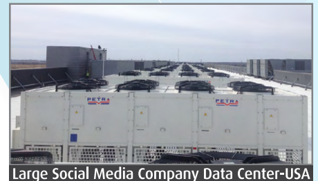
Large Social Media Company Data Center-USA
