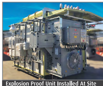
Explosion Proof Unit Installed At Site
