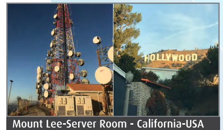
Mount Lee-Server Room - California-USA
