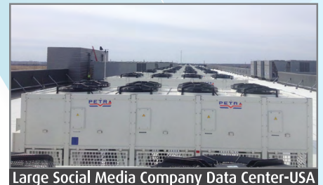
Large Social Media Company Data Center-USA
