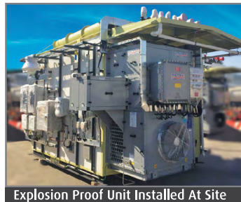
Explosion Proof Unit Installed At Site
