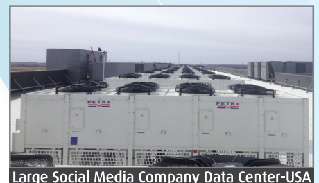
Large Social Media Company Data Center-USA
