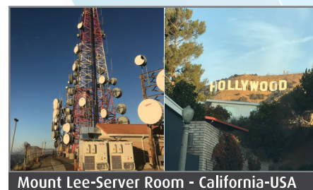
Mount Lee-Server Room - California-USA
