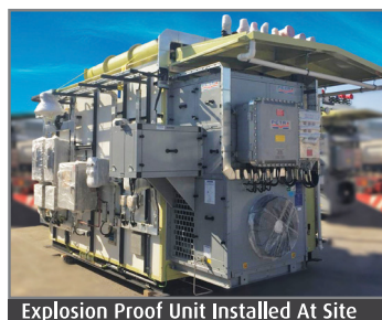
Explosion Proof Unit Installed At Site
