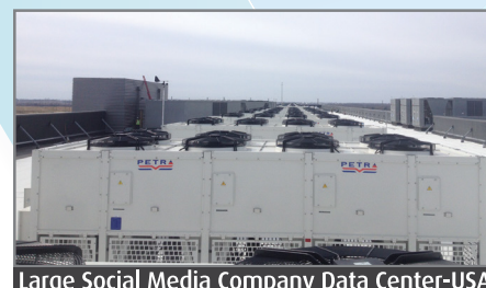
Large Social Media Company Data Center-USA
