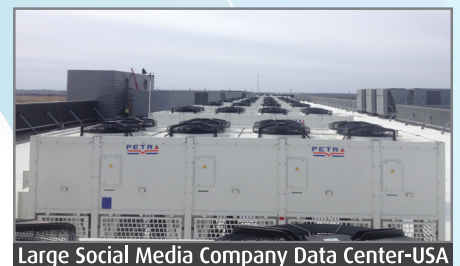
Large Social Media Company Data Center-USA
